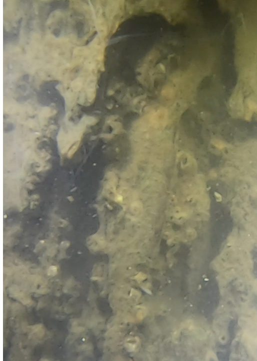
Photo 10: Pile erosion, Pier 32. It is possible this is from shipworms Teredinidae ; no worms observed but markings consistent with shipworm damage.
